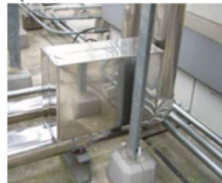
Used for the cooling towers A , B , and C
