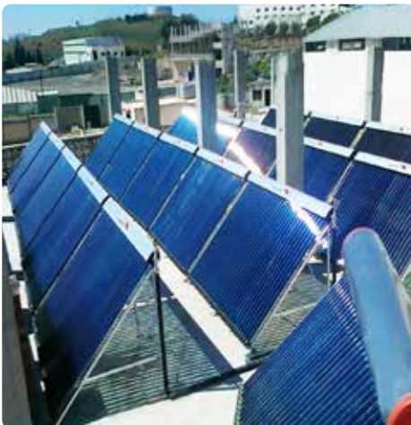
Solar heating panels of an apartment house.
