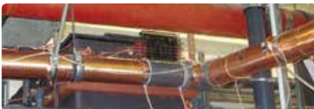
Vulcan S250 installed in the St. Joseph Hospital
