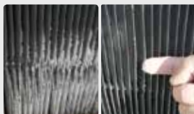
Cooling tower grids
