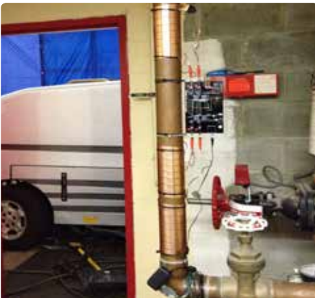
Vulcan S25 installed at Ice Land located in Hamilton, New Jersey
