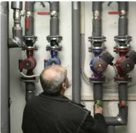
Piping system in an apartment building
